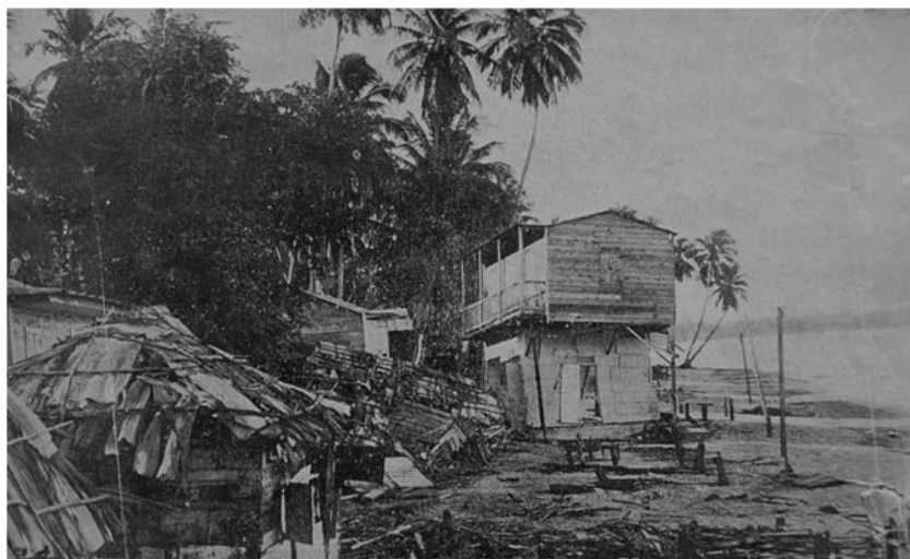
▲ Figure 4. Photo from Puerto Rico Ilustrado number 452, showing shoreline damage near zone 3 in Figure 2.
